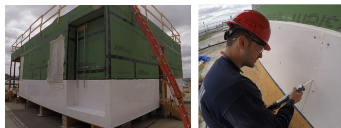
...with flood-proofing added in a layer on the underside of the floor system and continuing up the lower portion of the wall exterior extending above the base flood elevation.
