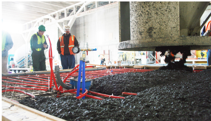
GCC precast wall panels were poured at a local plant showing that this technology is feasible now.
